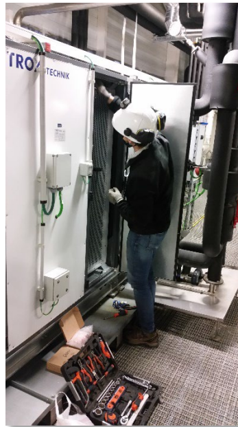
SMS installed on Conditioning Turbine inside the cabinet
